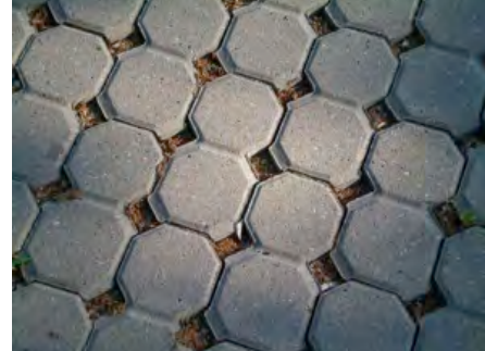
Figure 6: An Example of Porous Paving
