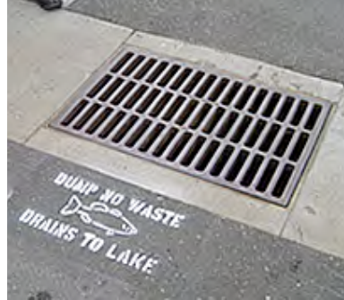
Figure 4: Storm drain marking
