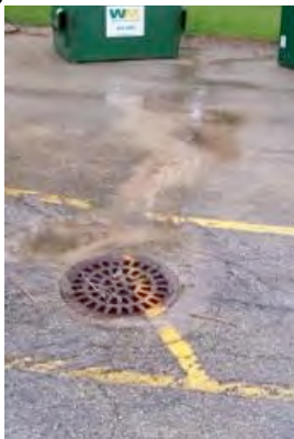
Figure 2: Rain water runoff
