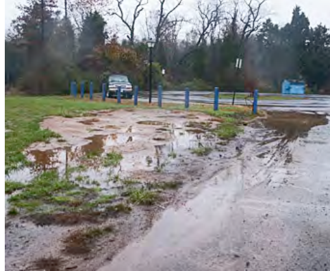
Figure 12: Displaced rain water runoff
