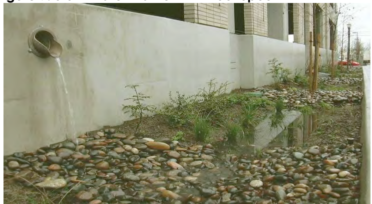
Figure 7: Stormwater Planter with Roof Spout
